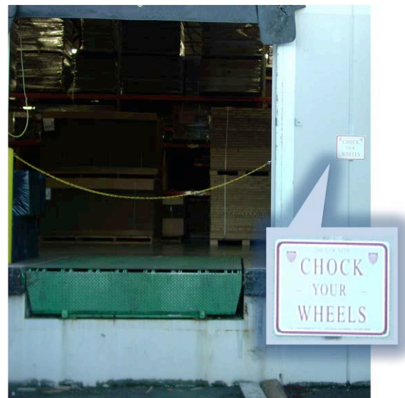
The dock involved in the incident where the driver was crushed (with “Kelly” dock plate). The white sign with red letters at right (shown enlarged) reads “chock your wheels.”
