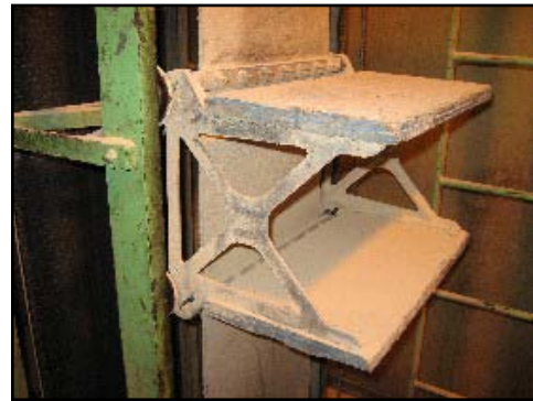
A close-up view of a platform step on the manlift shows the metal framework on the left and emergency ladder on the right.
