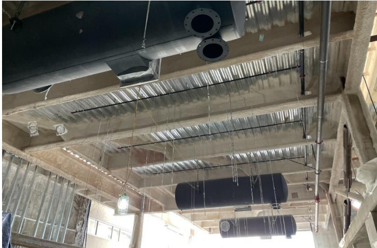
04/29/24 – Emergency generator mufflers suspended above level P3
